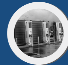
充电桩 Charging Pile
